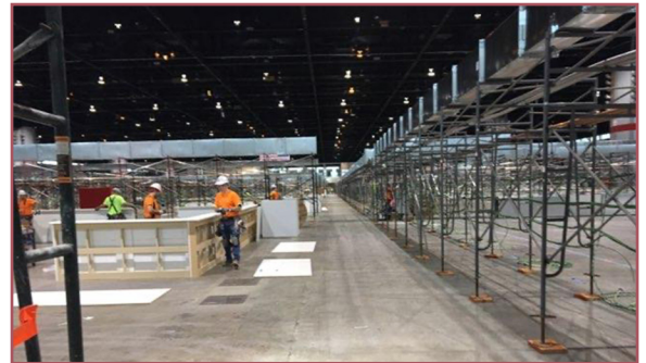
Construction crews work at McCormick Place to convert the convention center into a makeshift hospital.
