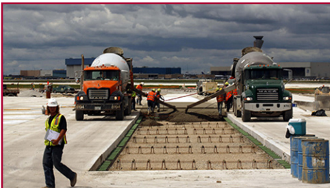
Construction work continues on a new cargo facility in the northwest corner of the airport while plans were announced that will build nine new gates and two new hotels.
