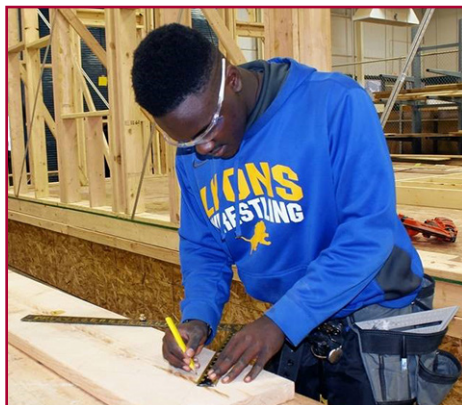
Jerry Presley, a senior at Lyons Twp. High School, uses a carpenter's square to mark out the cuts. Presley is in the construction trades program at TCD.
